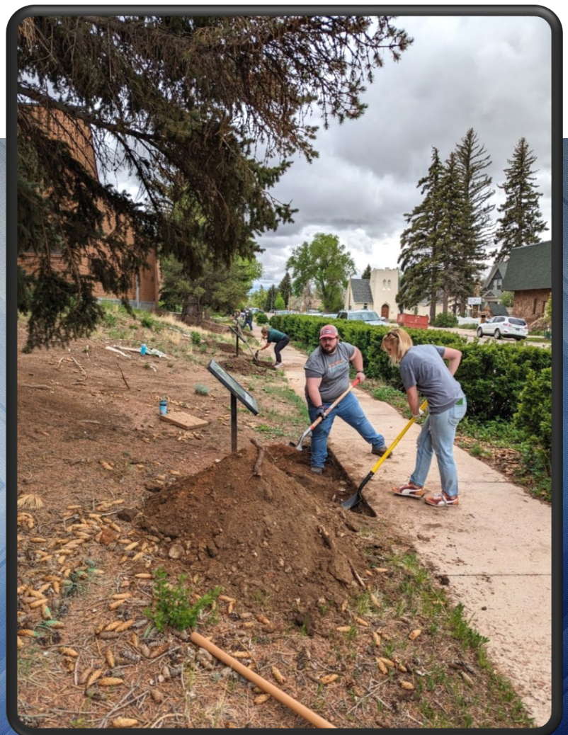
Workers dig areas for new cement pads along the story walk trail.
